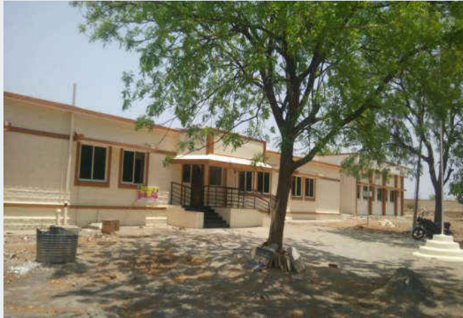
Construction of Wards, Mortuary Room, Toilets, renovation of existing OT and Labour room, providing ACs, Solar Lights, Furniture, DG set, Ambulance and medical equipment at Primary Health Centre, Mahagaon Cross, Gulbarga
